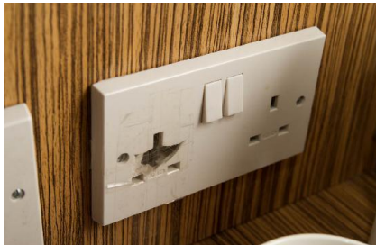
Cracked & chipped power socket
