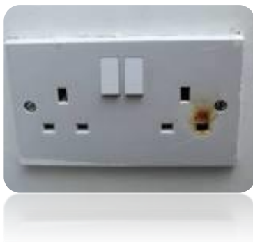
Burnt/charred power socket – this would indicate overload
