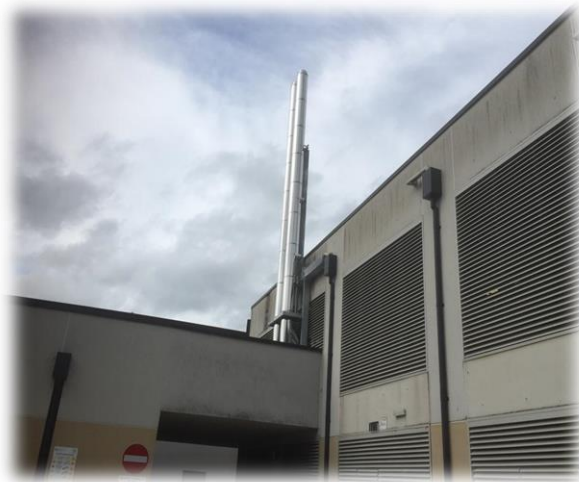
New external flues for the new dual fuel boilers at Ysbyty Cwm Cynon
