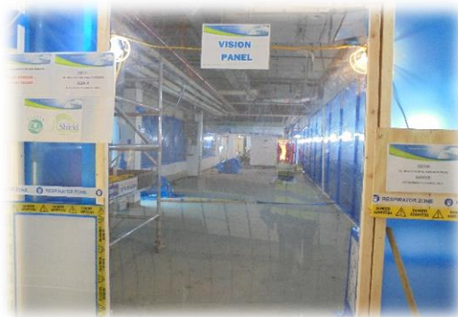
PCH Phase 1B works vision panel into a controlled Asbestos area
