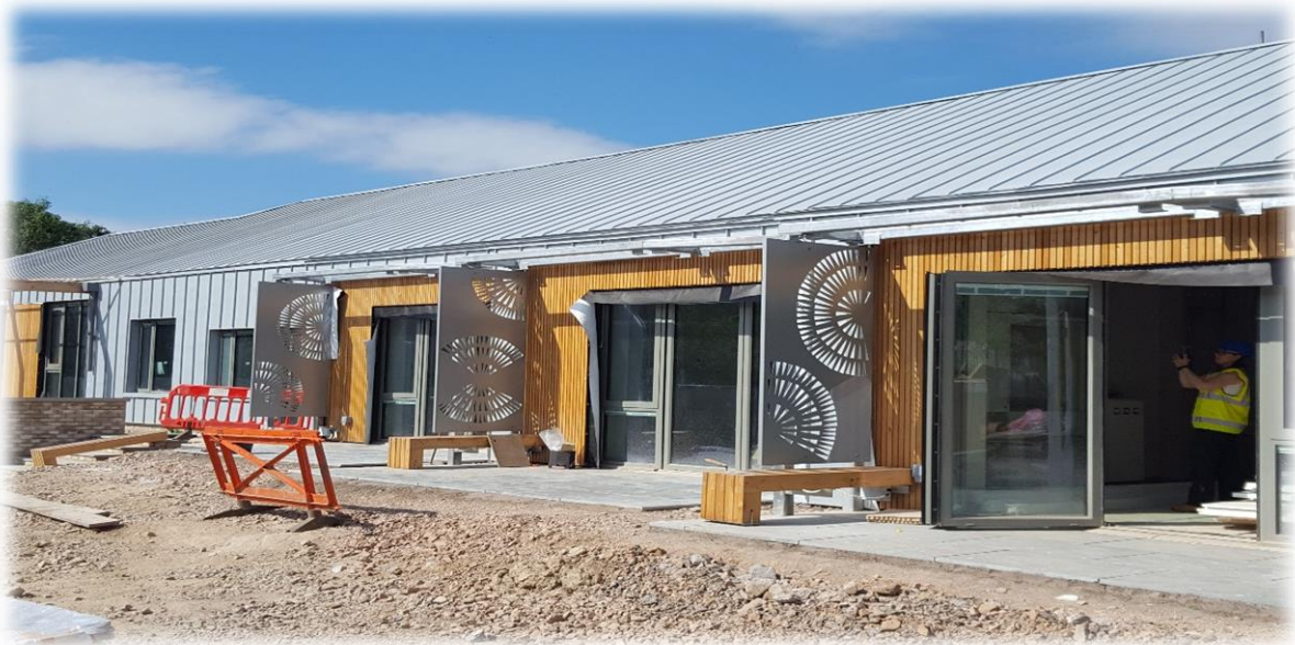
Exterior view of Y Bwthyn in construction at The Royal Glamorgan Hospital
