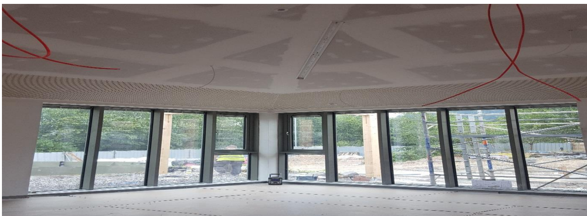
Interior view of Y Bwthyn in construction at The Royal Glamorgan Hospital
