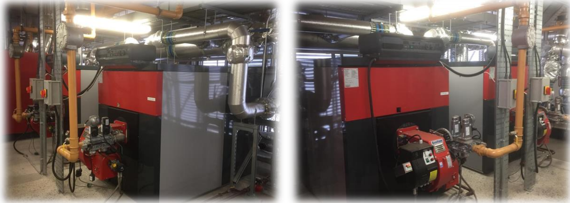
New dual fuel (gas & oil) boilers at Ysbyty Cwm Cynon to increase site resilience
