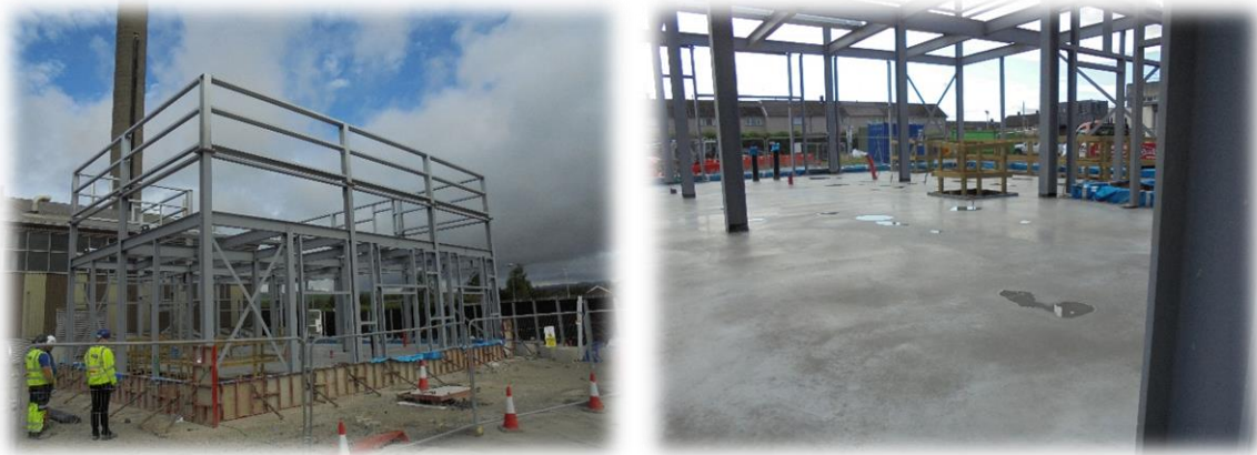
PCH Phase 1B steel work for a new plant room adjacent to the boiler house
